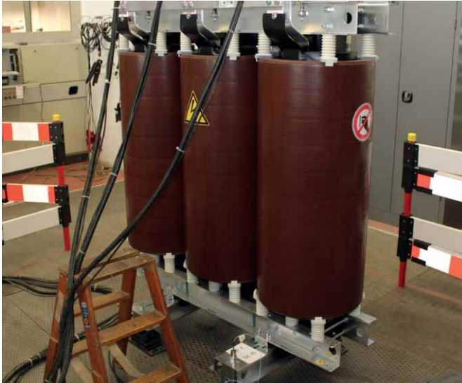
1000 KVA transformer in the testing laboratory
